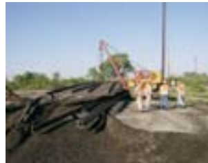
Maintenance of Way employees coordinate the installation of a new track panel on Track No. 627.
