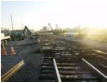
Rails and ties are removed to extend a track that will accommodate unit BNSF Crude Oil trains.
