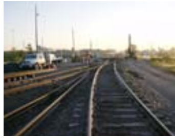
The installation of new rail is carefully planned, with everyone involved on the same page.
