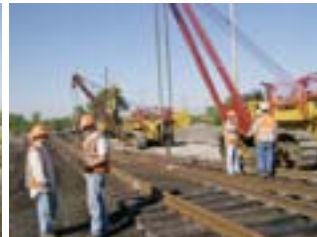
Employees conduct job briefings before they shift gears to a new aspect of the extension of Track No. 627.
