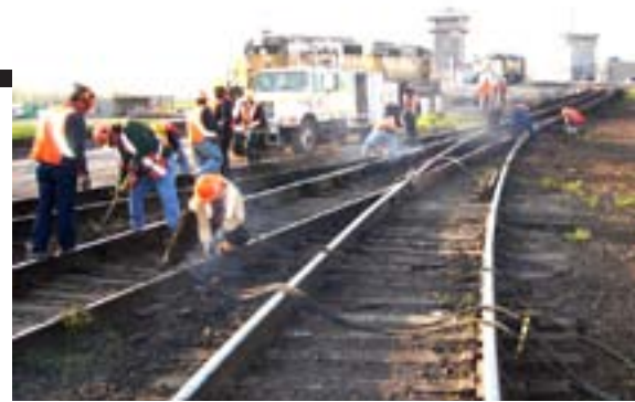
Working in close collaboration with other departments, Engineering employees focus on safely and efficiently completing various capital improvements in 2012.
