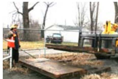
Sal Maloata, machine operator, left directs the placement of a plank on which Engineering material will be stored.
