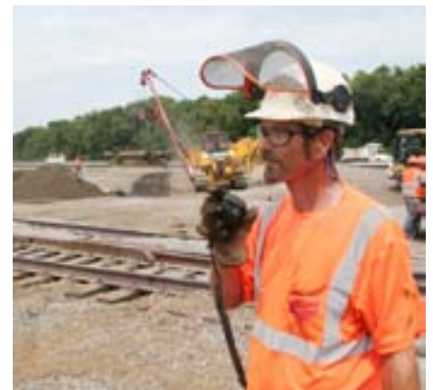
Steve Williams, foreman, radios a co-worker to ensure all employees are aware of their surroundings as Tracks 129 through 133 are extended.
