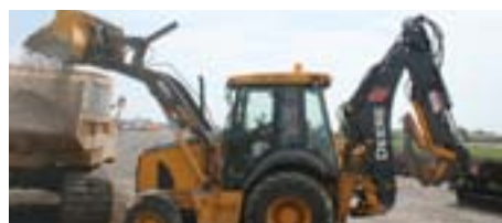
A front-end loader fills a dump truck with ballast to be spread on new track panels to facilitate construction.
