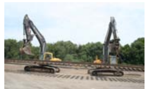
Cranes carry joined track panels into position to be attached to extend one of five tracks to greatly increase storage capacity at the east end the A&S yard.
