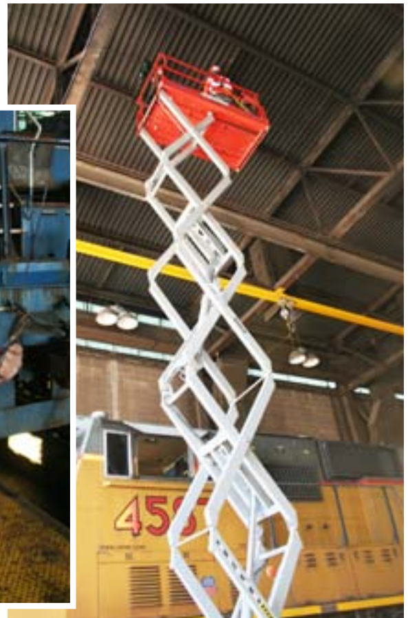
Jeff Pratt, signal foreman, works high atop the scissor lift to install new lighting in the car shop and roundhouse work areas.
