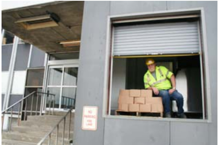
Jim Shewmaker, foreman, inspects cases of water bottles on a pallet placed in the storage room directly by forklift after a new overhead door was installed near the General Office Building entrance.
