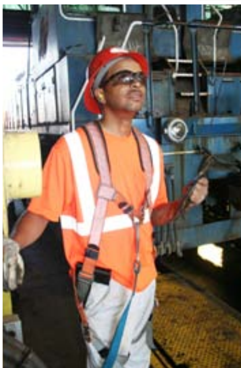
Adrian Abernathy, signalman, watches his co-worker on the scissor lift while feeding wire to him as new lights are installed.
