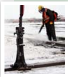
Ice and debris can clog switches in the wintertime. It's important for employees to report switches that are hard to throw.
